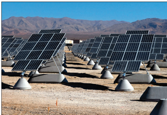
Figure 1.8 A power plant at Nellis Air Force Base utilizes photovoltaic solar cells. Stocktrek Images/Getty Images
